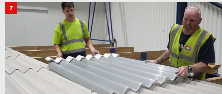
Place the first sheet on top of the fibre cement sheets whilst using a small fibre cement jig to ensure that the Heatguard 50 sits truly square when laid.
