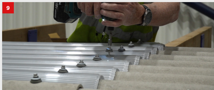
The primary fixings must be secured first and fixed into every corrugation peak.
