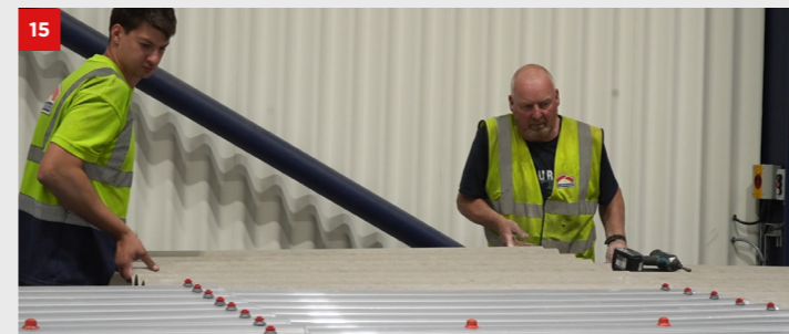
Similar to the first run, the last run should be laid using fibre cement sheets and fixed in accordance to the design guide.
