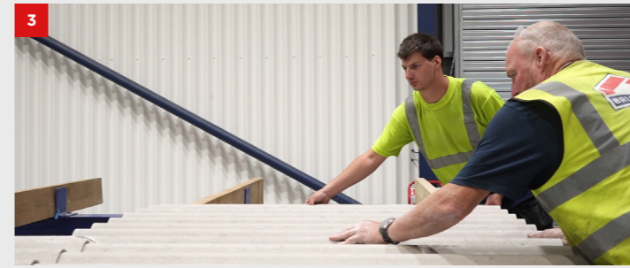
Once you have laid the first run, the first sheet of the next run should be our Big 6 fibre cement profiled sheeting.
